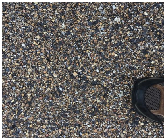
FIGURE 5 Minor between-wheelpath longitudinal cracking in S2.
