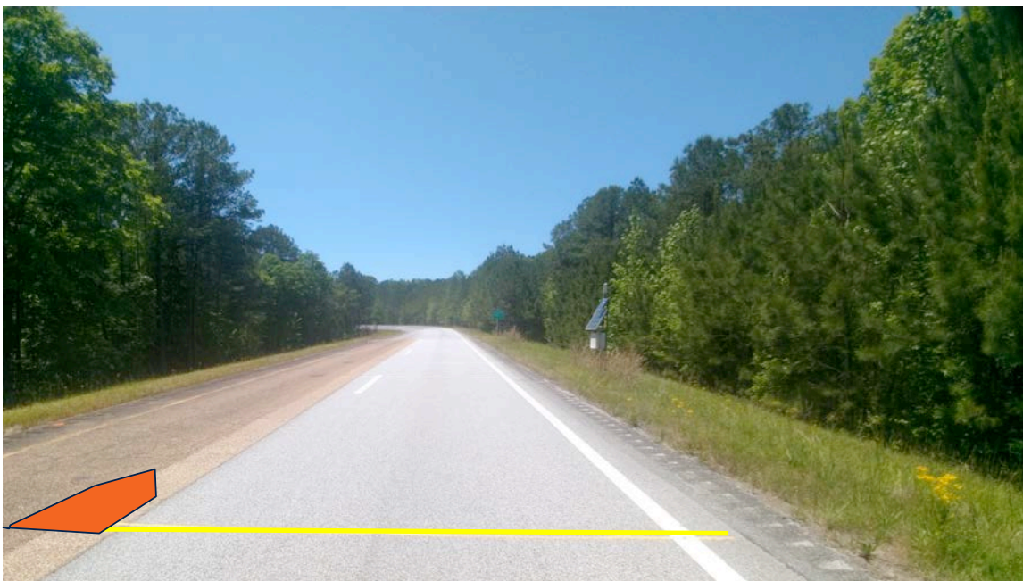
FIGURE 17 Subsection N13-B ARGG, 0.35-inch rutting, 3.1% cracking (April 2024).
