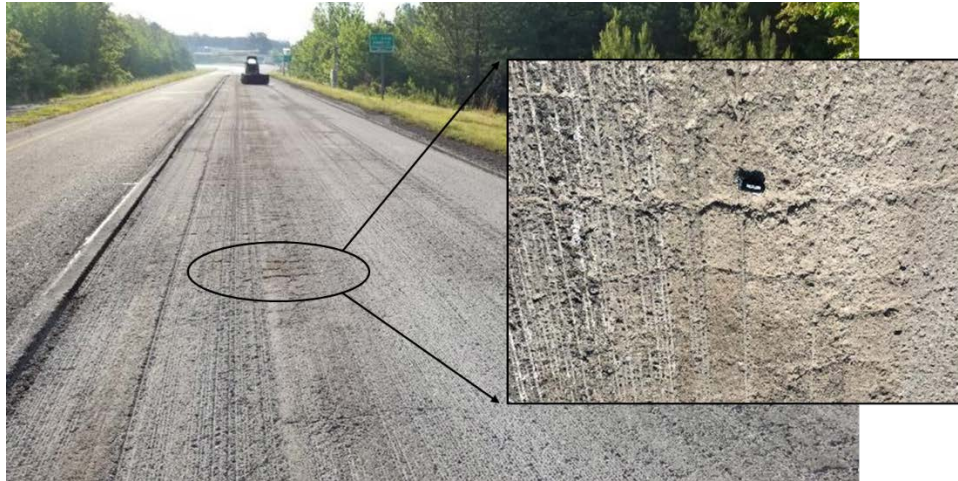
FIGURE 2 Fatigue cracking in underlying pavement of Sections 10 and S11 after milling.
