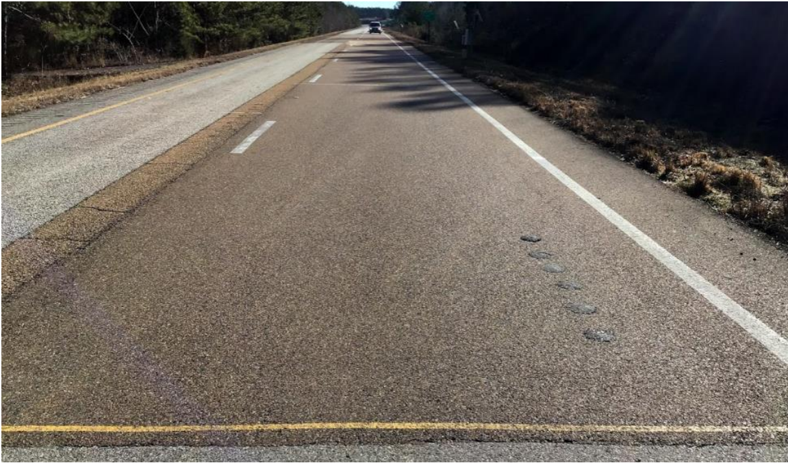
FIGURE 2. Test Section S2 near the end of first trafficking cycle.
