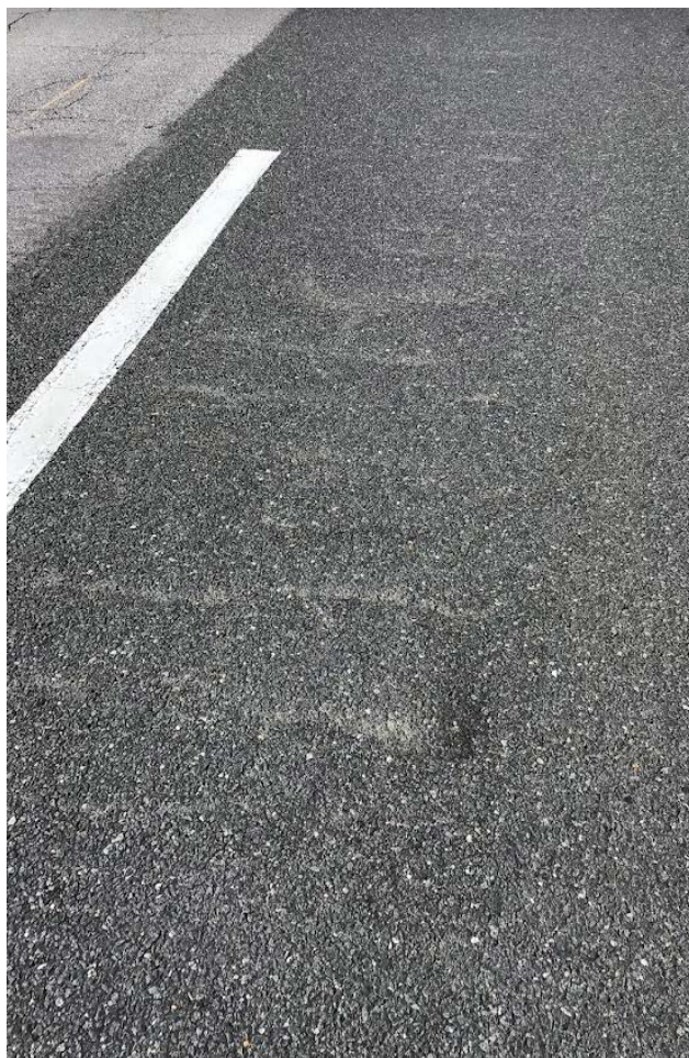
FIGURE 3 Wheelpath fatigue cracking in N4 on 1/22/2024 (39.1 million ESALs).
