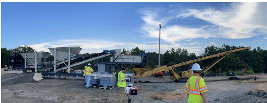
FIGURE 3 Pugmill Systems portable pugmill.
