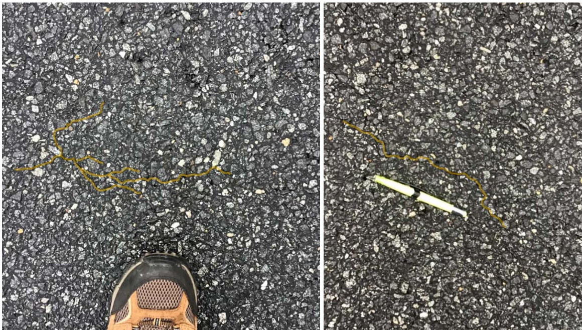
FIGURE 2 Sample cracking in N4 on 1/25/2021 (29.6 million ESALs).
