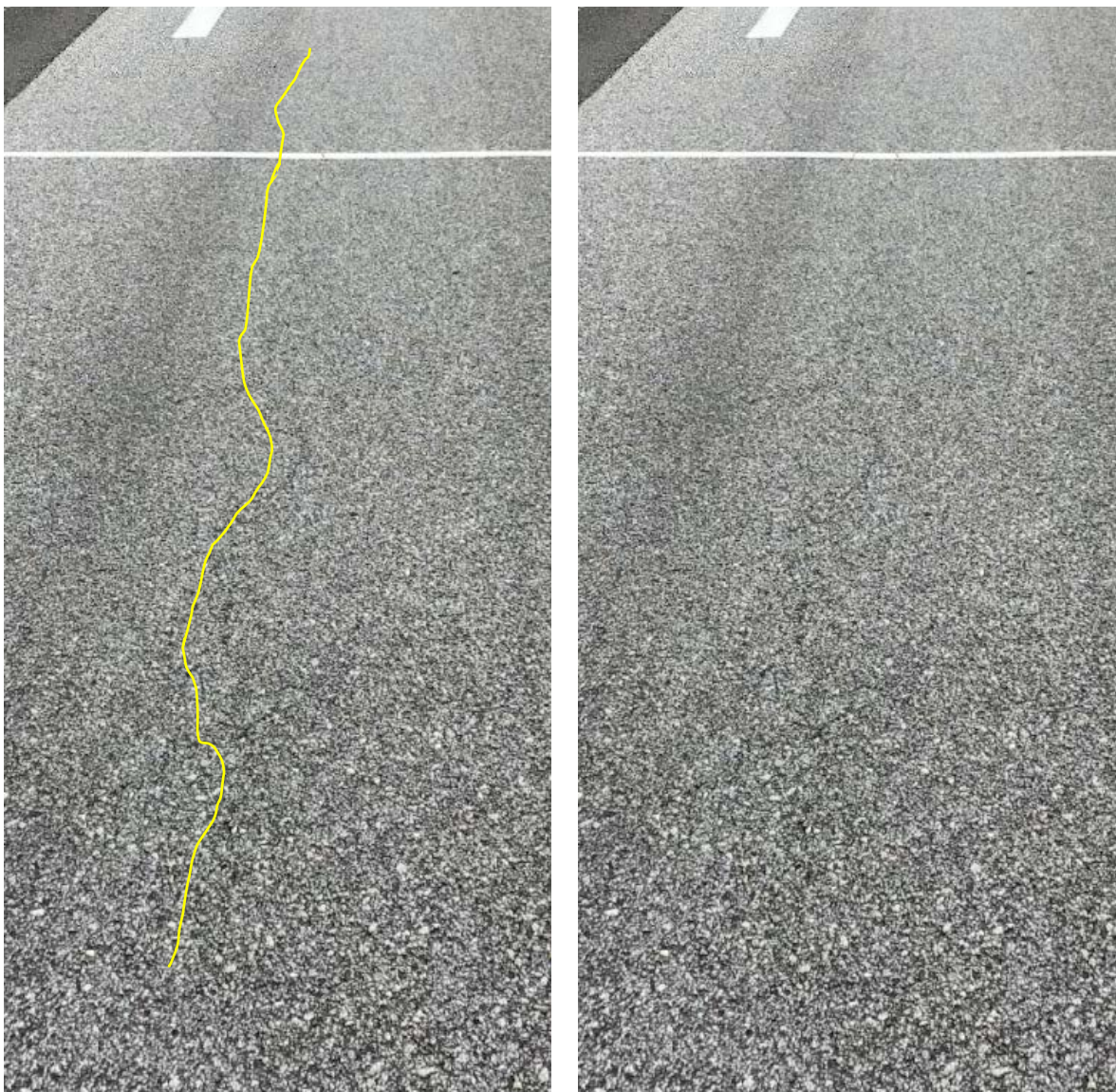
FIGURE 6 Longitudinal crack at edge of inside wheelpath in S9 at end of second test cycle (with and without highlighting).
