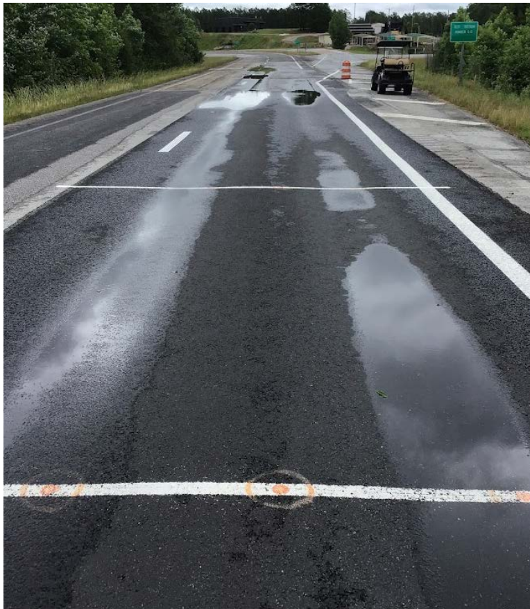
FIGURE 6 Rutting in Section S12 (April 2022).
