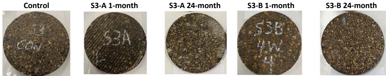
FIGURE 3 Section S3 pavement surfaces 1 month and 24 months after treatment application.
