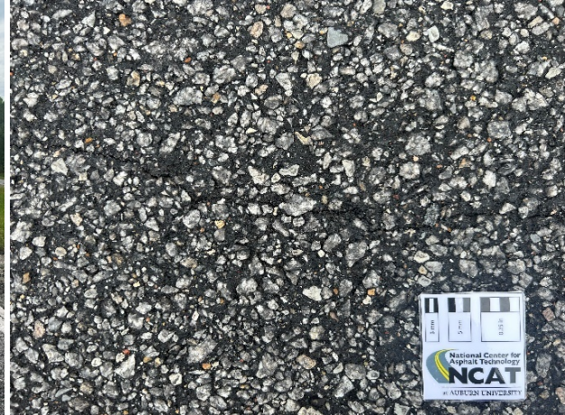
E6A (87.8% of G_{mm} ) representative cracking
