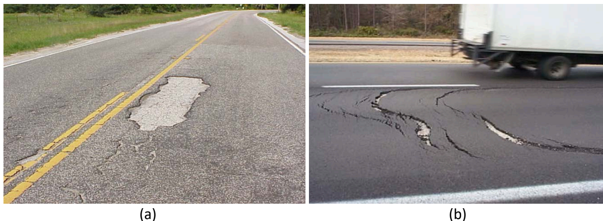
FIGURE 1 (a) Delamination and (b) slippage cracking (2).
