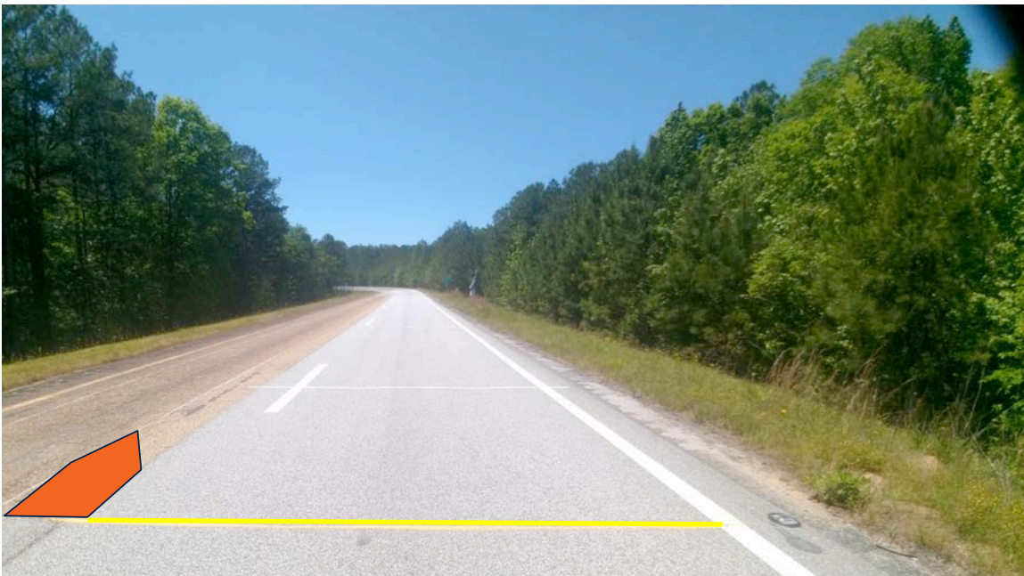
FIGURE 16 Subsection N13-A RAP chip seal, 0.41-inch rutting, 0.8% cracking (April 2024).
