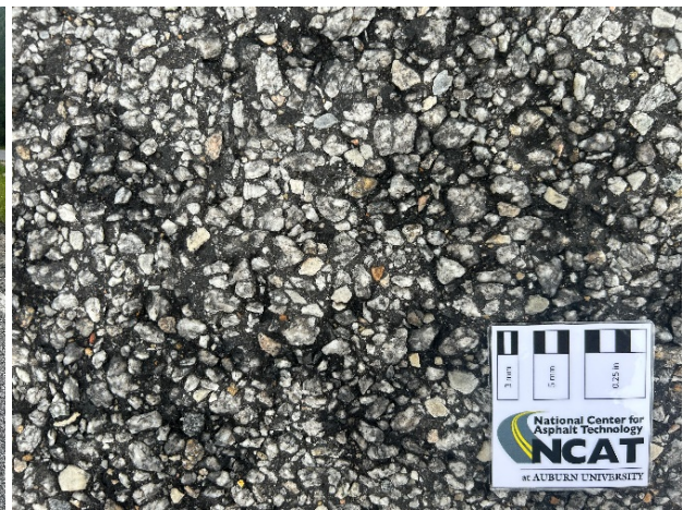
E5B (92.0% of G_{mm} ) representative cracking
