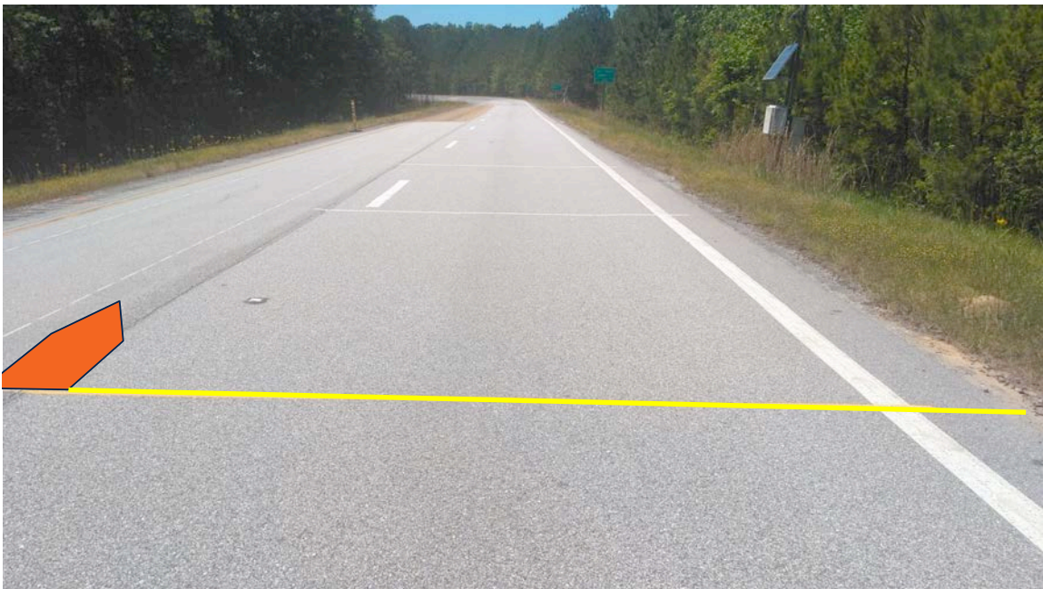
FIGURE 14 Subsection N12-B PETROMAT ® , 0.27-inch rutting, no cracking (April 2024).
