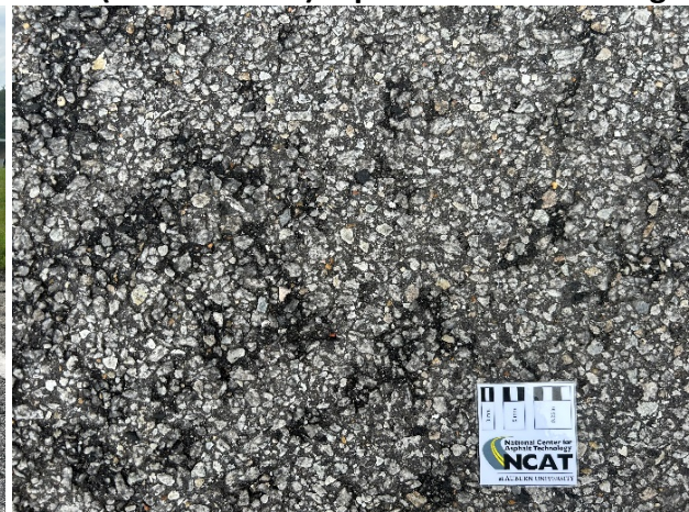
E6B (89.7% of G_{mm} ) representative cracking
