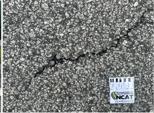
E5A (93.6% of G_{mm} ) representative cracking
