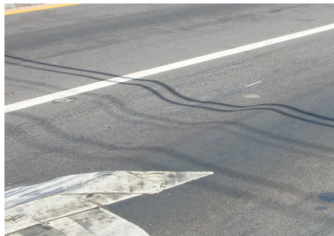
Figure 14. Example of rutting on a high traffic road.
