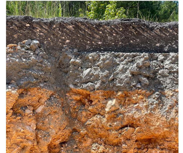
A cross section taken prior to construction showing the Test Track subgrade (bottom), aggregate base (middle) and hot mix asphalt overlay (top).
