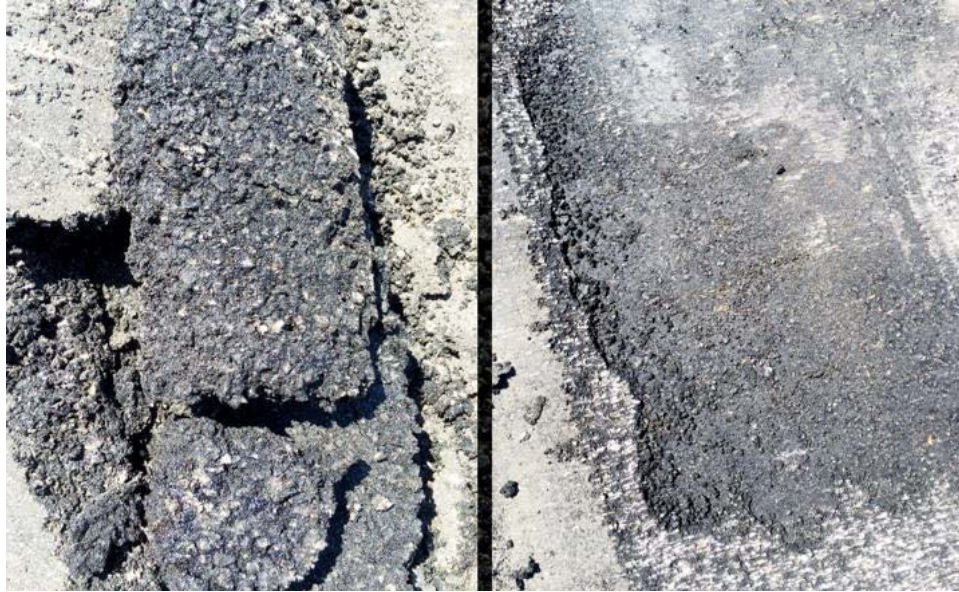
Figure 4 Interface Between Layers in Failure Area
