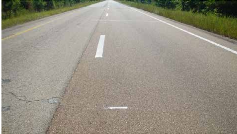
Figure 2 Crack Observed in Section S3 Near the Inside Edge of the Outside (Research) Lane
