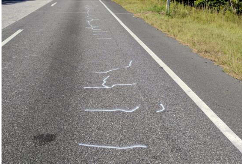
Figure 10. Mapped Cracks on the Test Track
