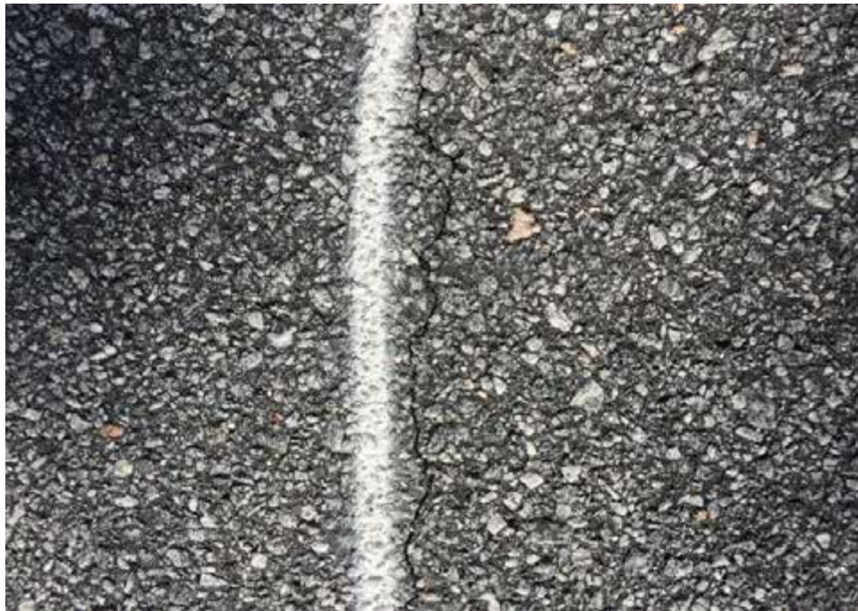
Figure 6 Low Severity Cracking in N12
