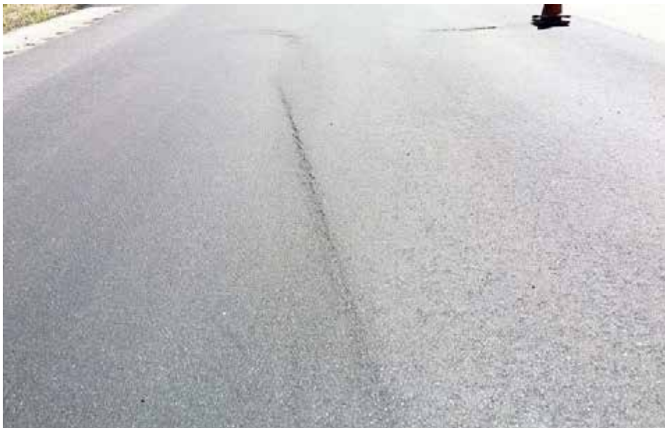
Figure 3 Slippage Failures of Section N7 After Repaving
