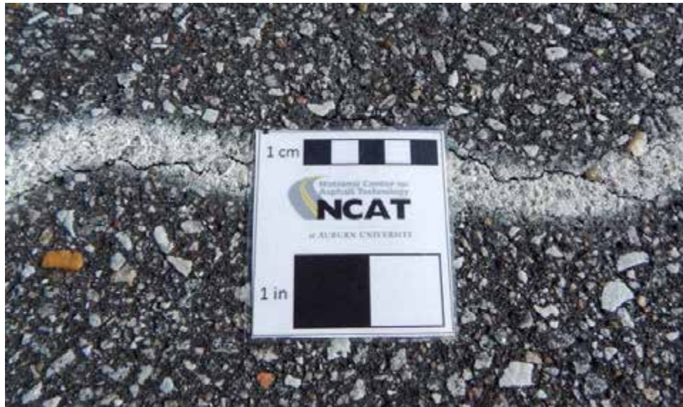
Figure 19 Close-up of Hairline Cracks in Sections N7 and N1
