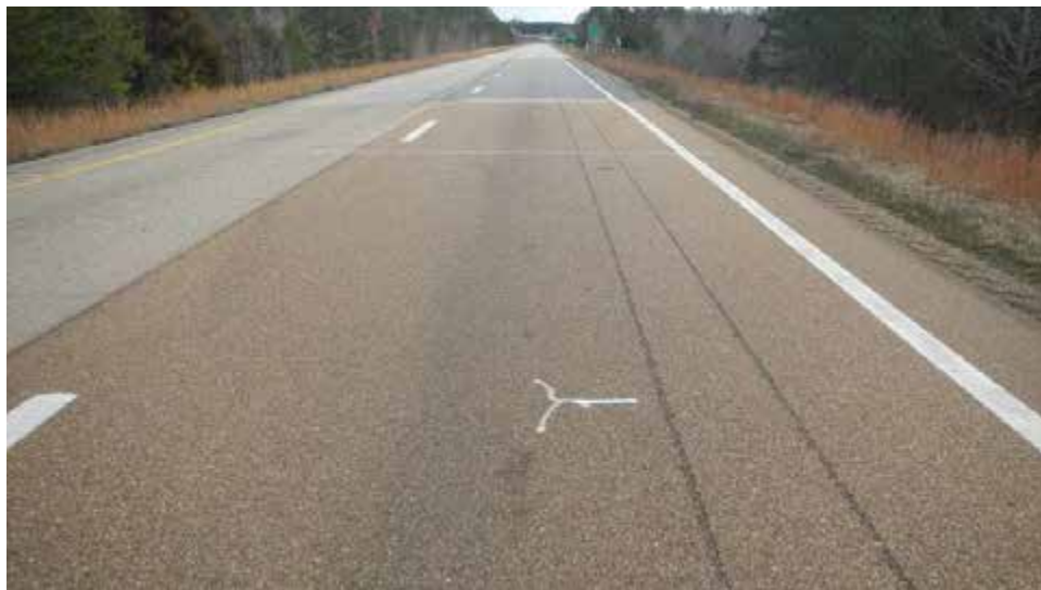
Figure 3 Crack Observed in Section S3 Near Center of the Outside (Research) Lane
