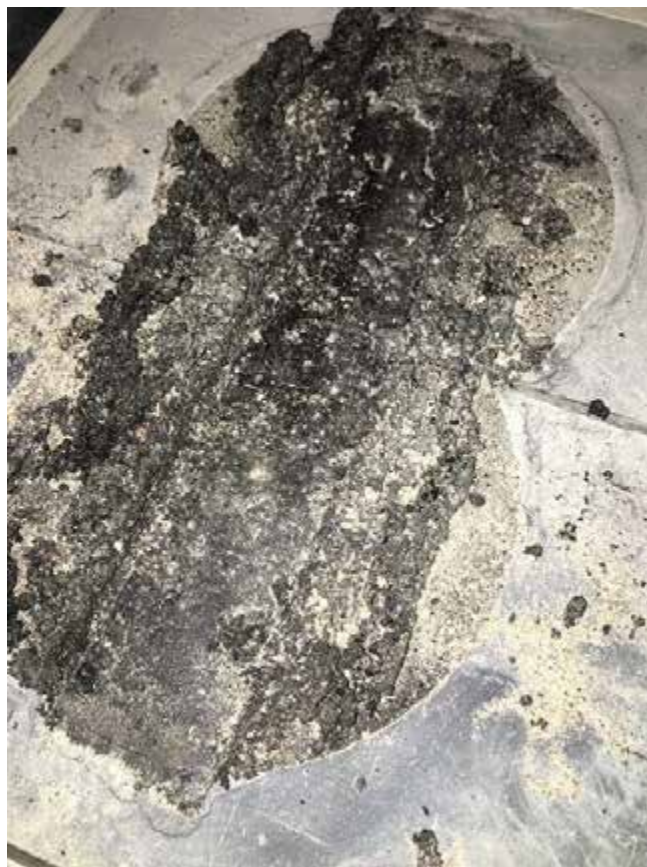
Figure 4 Calcined Bauxite SMA Mixture Stripping Failure
