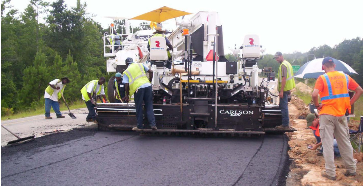
Figure 1.3 Paving the Surface Layer of a Test Section on the 2009 NCAT Test Track
