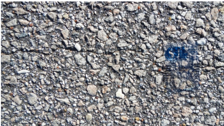
Figure 3.6 Close-up Photograph of Section E5 Showing Texture and Crack
