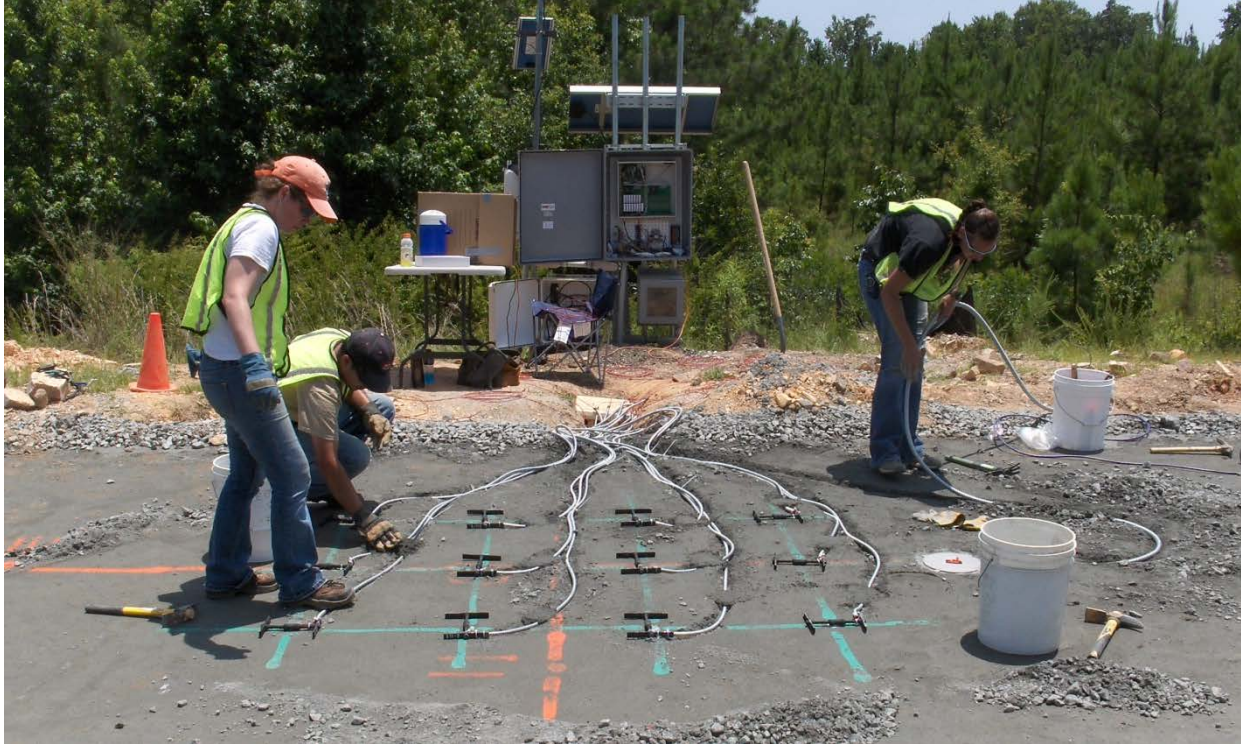
Figure 1.2 Installation of Strain Gauges and a Pressure Plate Before Placing the Asphalt Base Course
