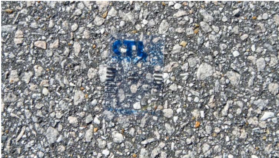
Figure 3.5 Close-up Photograph of Section W5 Showing Texture and Hairline Crack Just Below the Scale
