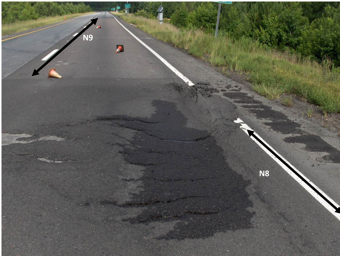
Figure 3.2 N8 Pavement Failure after Conventional Mill and Inlay
