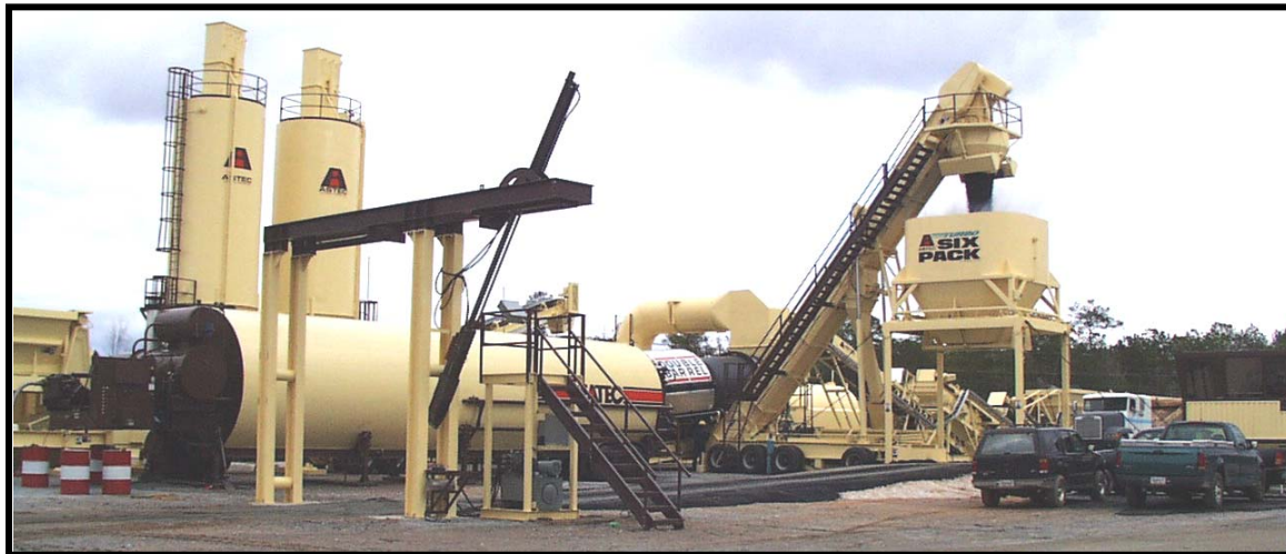
Figure 2. Onsite Double Drum Asphalt Plant Used to Produce All Track Mix
